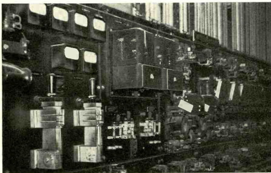
Relay panel which controls section motors and transfers them from starting generator to running generator. Board is about 7 feet tall and 20 feet long.
